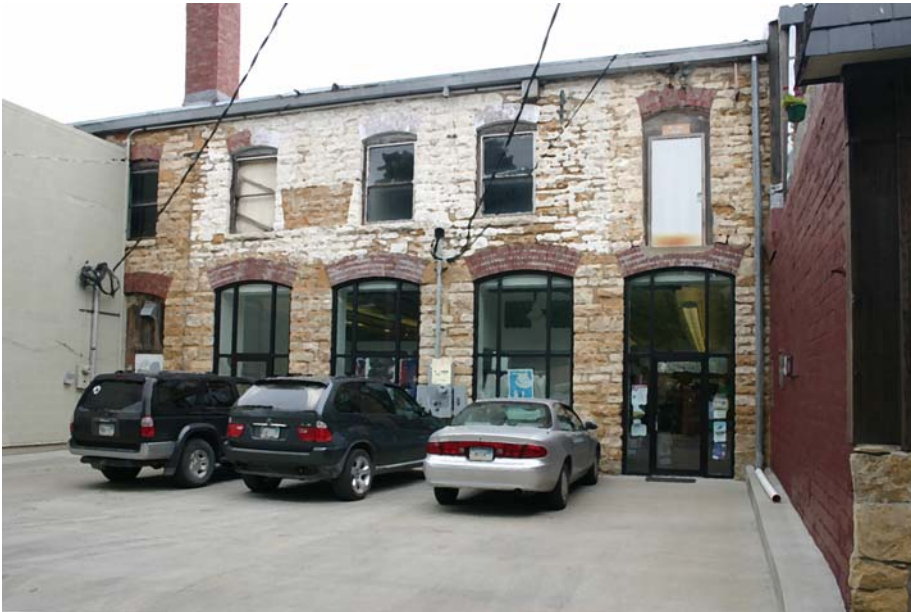
In this example, appropriate modern treatments have been applied to enhance and introduce a series of entryways, but the original upper story windows have been unsympathetically altered.
