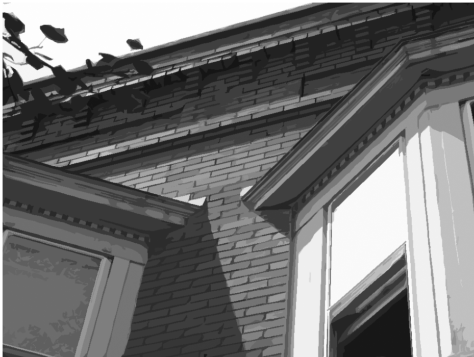
Brick, wood, stone, terra-cotta, and cast iron are typical for Downtown Lawrence.
