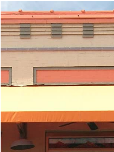
Details such as brick corbelling, raised belt courses, or inset panels should be retained.
