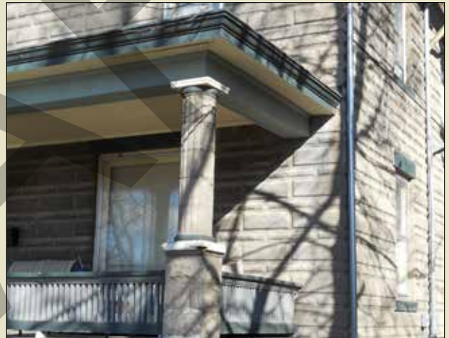
The load being supported by the columns should be expressed in the design of the structure. Columns and their bases should be evident.
