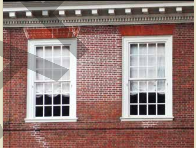
Unlike this example, walls should be repaired with like materials that match in color, texture, and construction method
