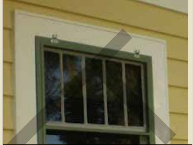
A good example of painted, wooden storm windows that are appropriate for this application.
