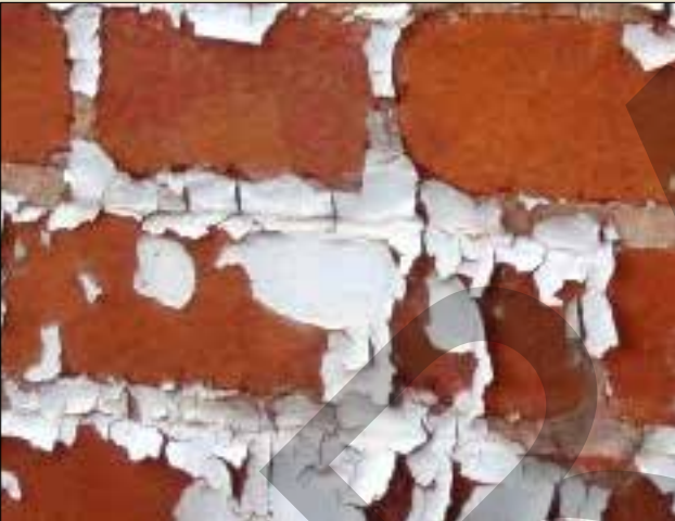
Masonry should not be painted.
