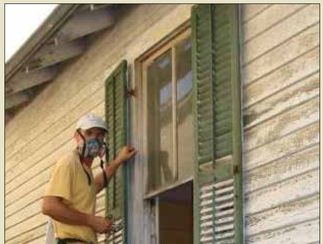
When replacing elements make sure they match the originals in proportion, scale, mass and materials.
