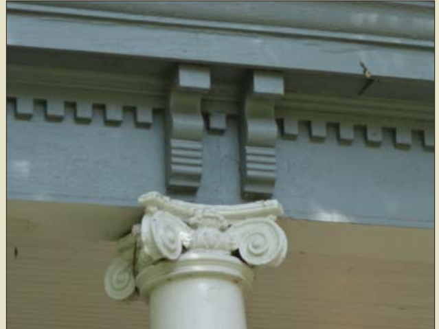
Porch details should be commensurate with the load they support, such as this example.
