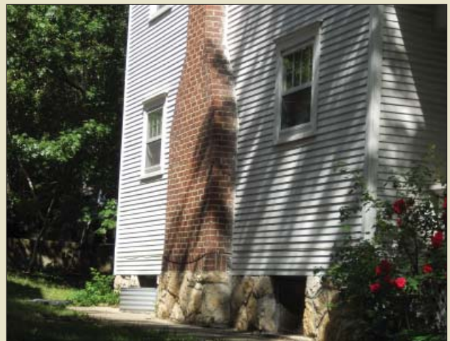
Original chimneys should be retained. If adding a chimney, do this on the back of the building so it's not visible from the street.
