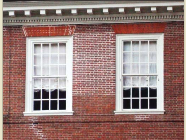
Unlike this example, walls should be repaired with like materials that match in color, texture, and construction method
