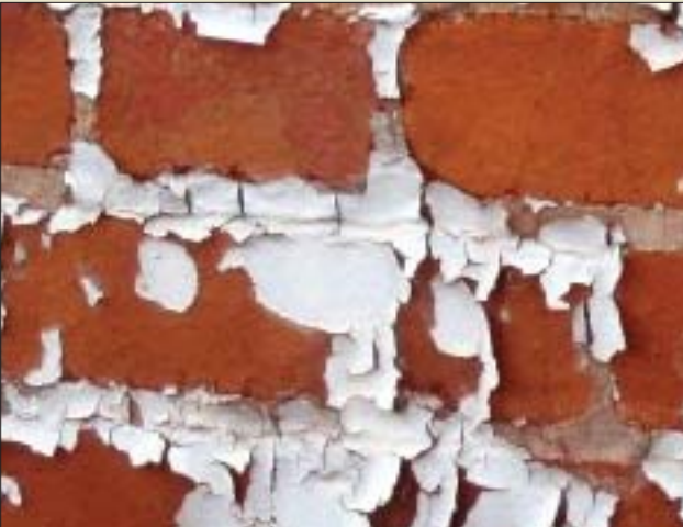
Masonry should not be painted.
