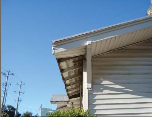
An unacceptable example of vinyl siding concealing original features.
