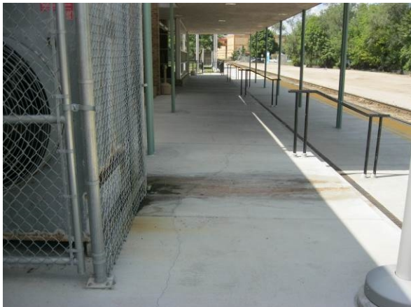
Photo #3 Image of staining observed on the concrete near the cooling unit.
