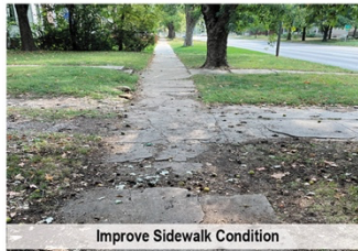
Improve Sidewalk Condition
