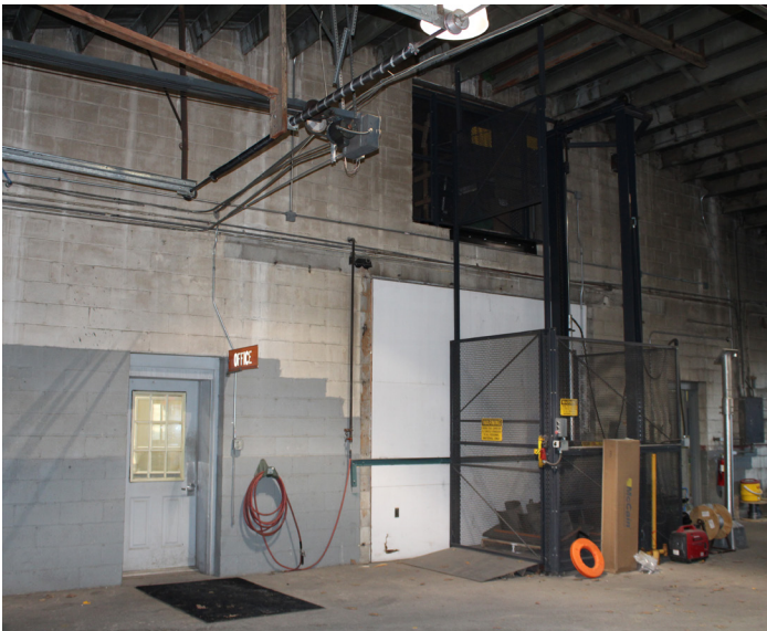
Concrete floors, partially painted CMU walls, exposed structure, water damage, poor condition
