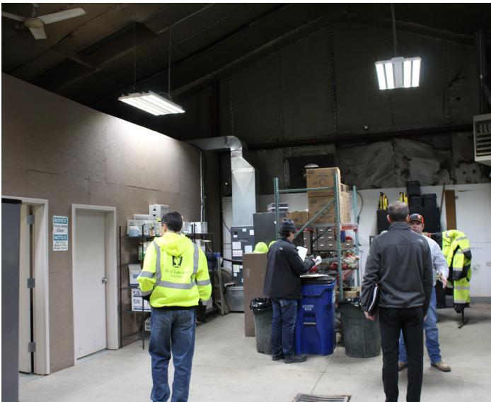
Concrete floor, damaged insulation, overall poor condition
