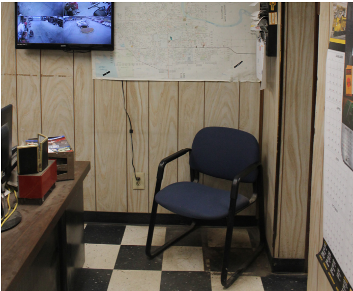
Linoleum tile floor decorative wall covering, poor condition
