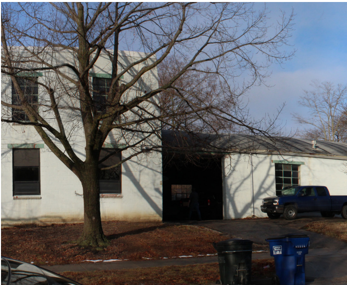
Exterior - poor condition
