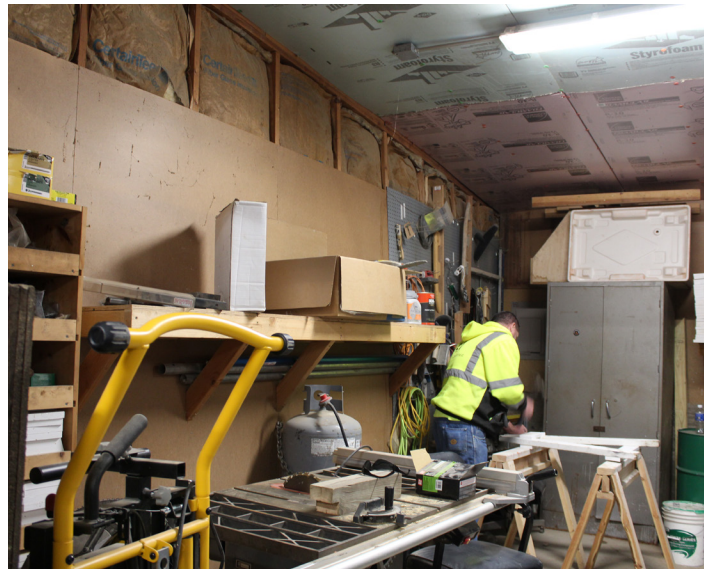
Concrete floor, exposed insulation, surface mounted fixtures, overall poor condition
