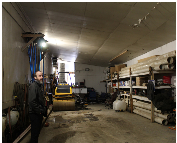
Concrete floor, ceiling damage, overall poor condition
