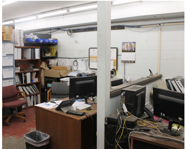
Concrete floor, painted CMU walls, gyp board ceiling, surface mounted fixtures, poor condition
