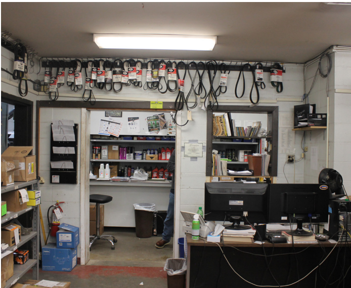
Concrete floor, painted CMU walls, gyp board ceiling, surface mounted fixtures, poor condition
