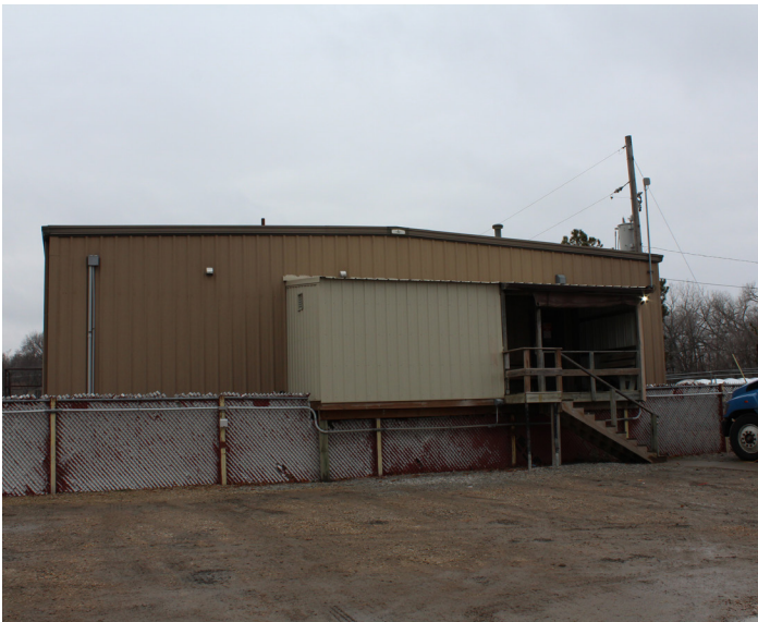
Exterior - poor condition
