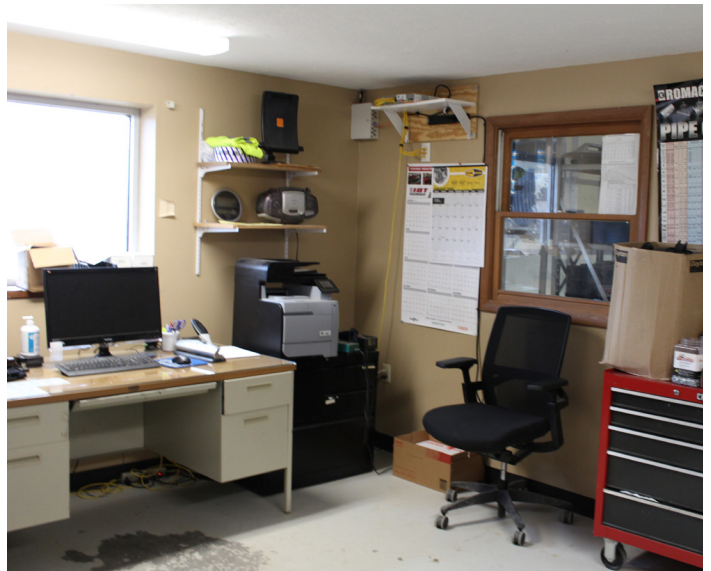
Concrete floor, painted gypsum board walls, ACT ceiling, poor condition
