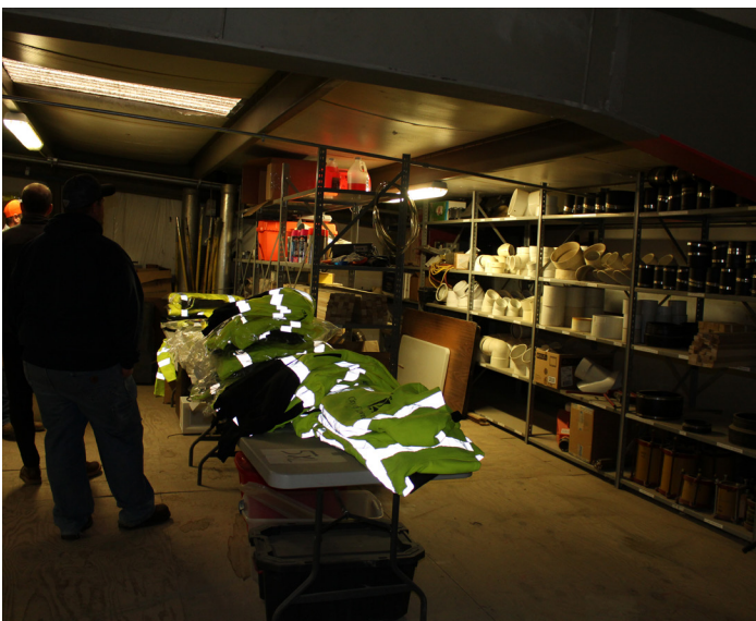
Concrete floor, steel structure, bag insulation, overall poor condition
