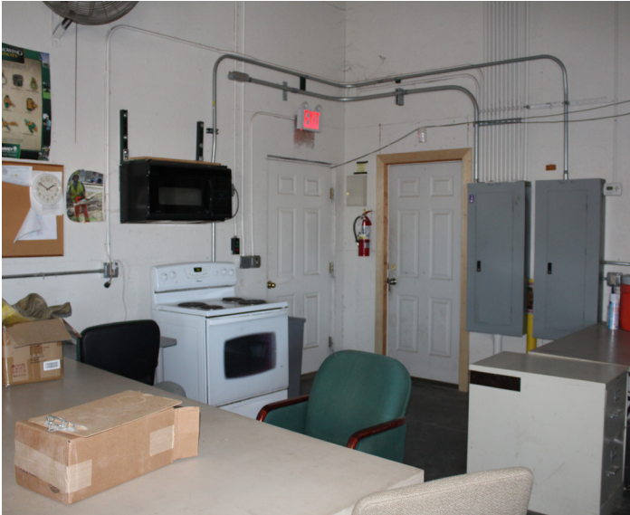
Concrete floor, gypsum board walls, poor condition
