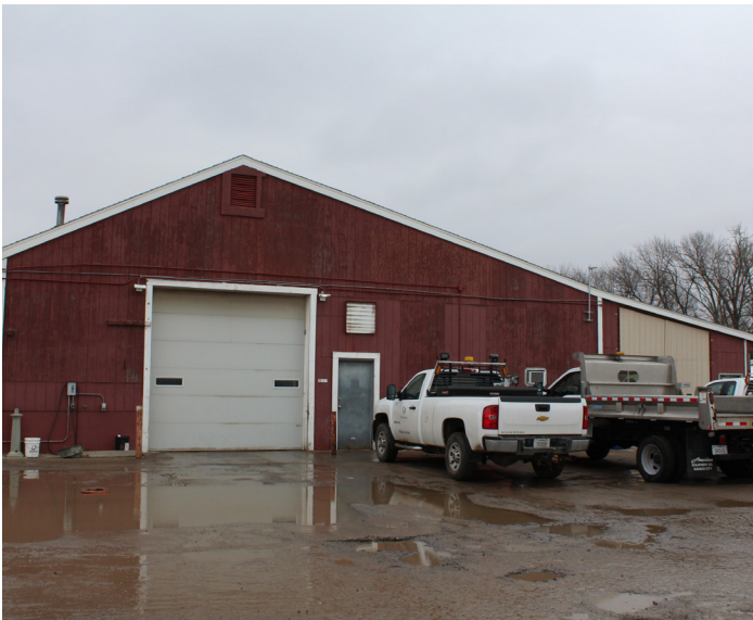
Exterior - poor condition
