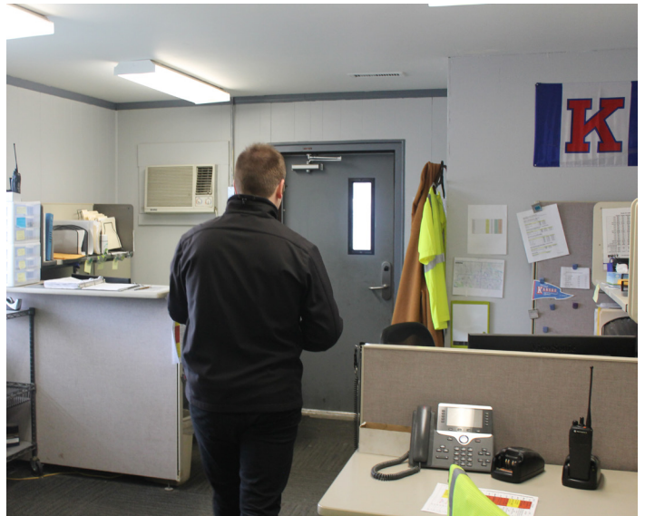
Carpet tile flooring, painted CMU walls, gypsum board ceiling, surface mounted fixtures, poor condition
