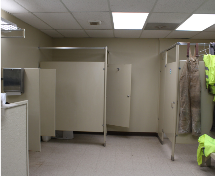
Linoleum flooring, painted gypsum board walls, ACT ceiling, poor condition
