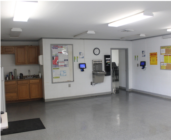
Linoleum flooring, painted CMU walls, gypsum board ceiling, surface mounted fixtures, fair condition
