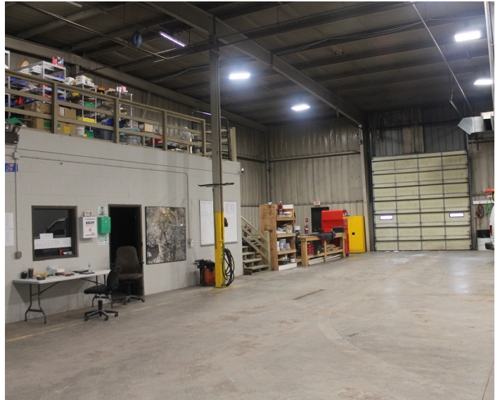
Concrete floor, exposed pre-engineered steel structure, poor condition
