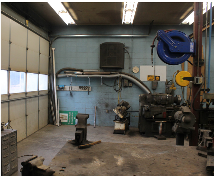
Concrete floor, painted CMU walls, surface mounted fixtures, poor condition
