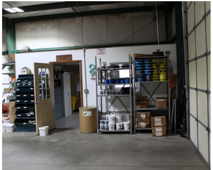
Concrete floor, damaged insulation, fair condition
