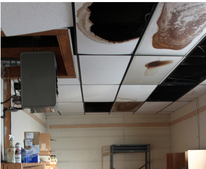
Water damage, poor condition
