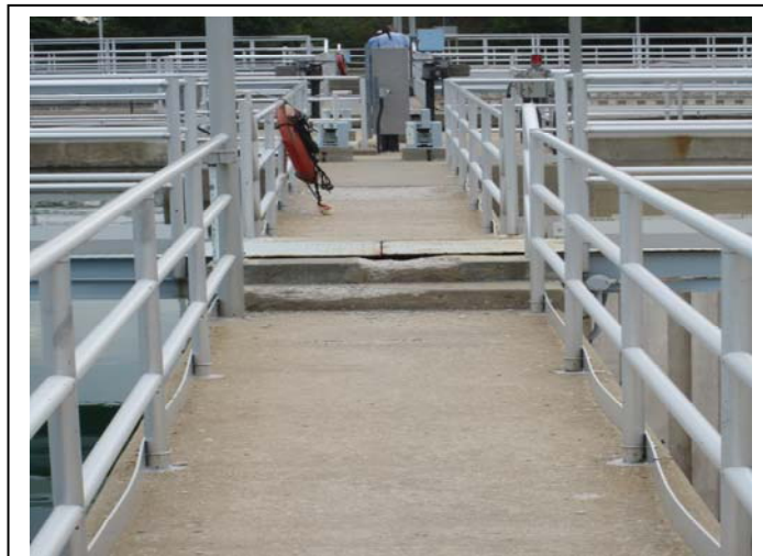
Item #3: Concrete walkway's stairs
