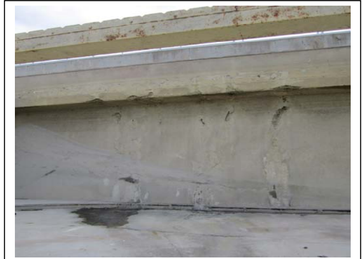
Item #6: Basin's Interior Wall Surface Degradation
