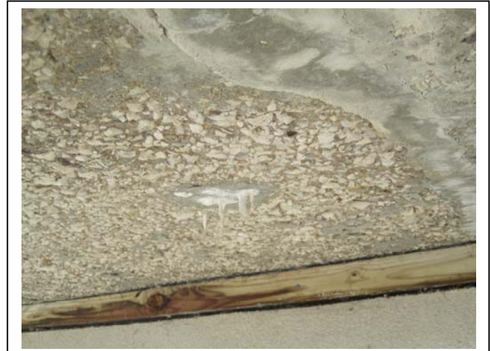
Item #5: Bottom of Primary Basin Trough's Base Slab
