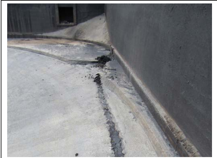
Item #1: Crack in Carbon Contact Basin's Base Slab
