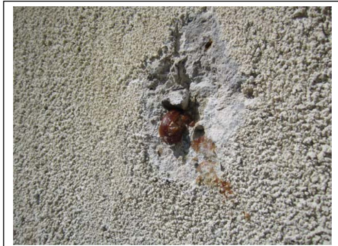
Item #7: Holes in Basin's North Wall
