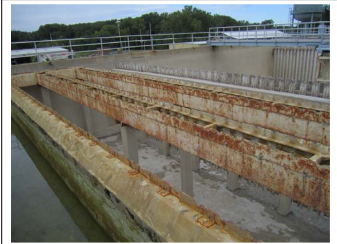
Item #8/9: Weir Trough/Plate's Rust and Connection
