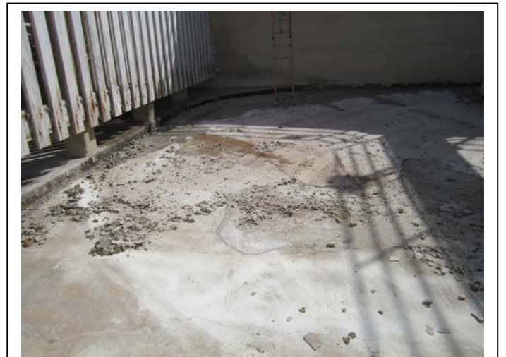
Item #5: Cracks in the Secondary Basin's Base Slab
