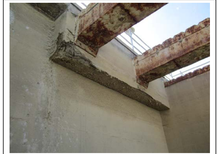
Item #9: Weir Troughs Rust and Connection
