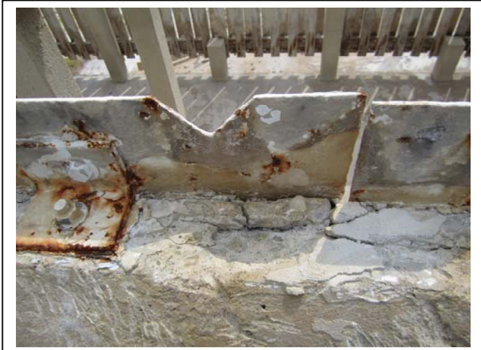
Item #9: Basin's weir plate to concrete connection.
