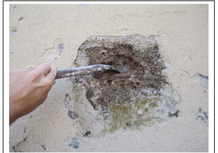
Item #7: Holes in Basin's North Wall
