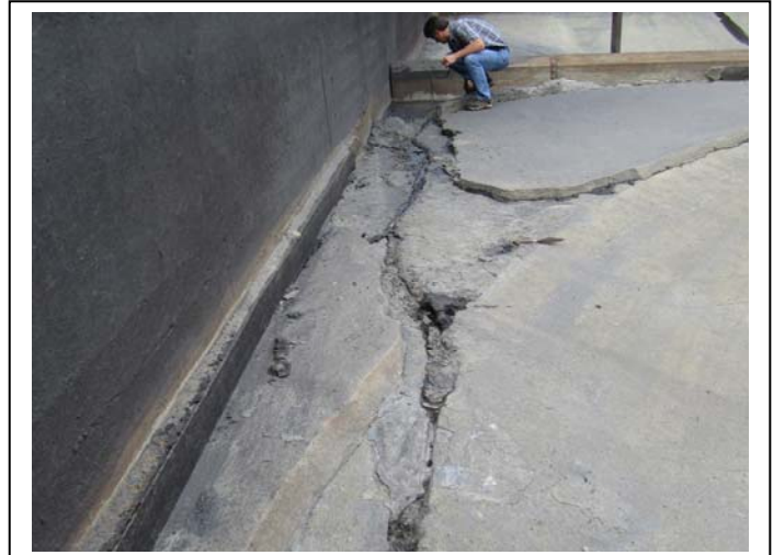
Item #1: Crack in Carbon Contact Basin's Base Slab
