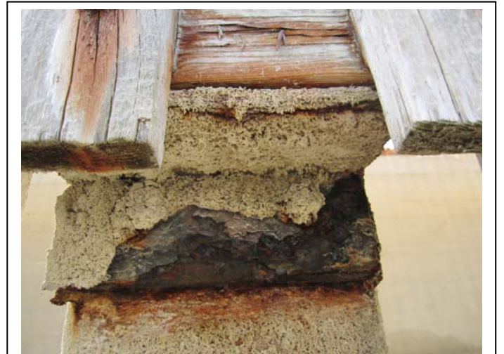
Item #11: Baffle Wall Degraded Metal Support Clip
