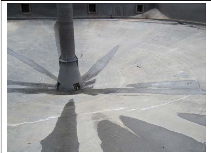
Item #2: Carbon Contact Basin's Slab Seepage
