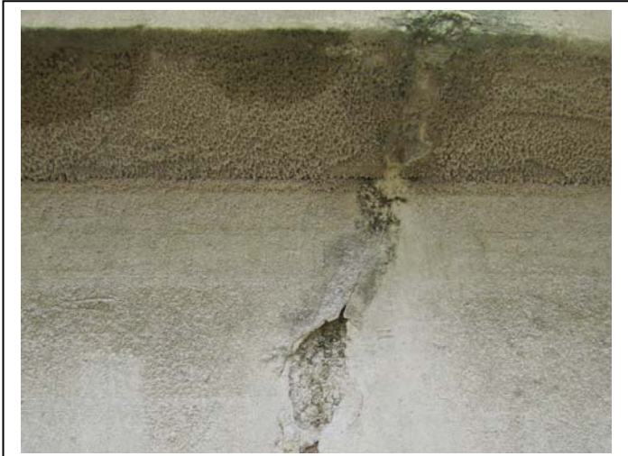
Item #6: Basin's Interior Wall Surface Degradation
