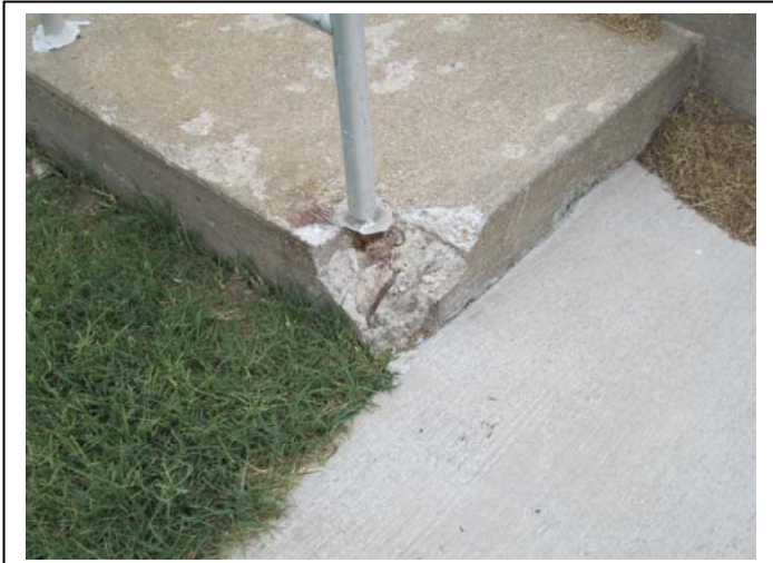
Item #1: Handrail to Concrete Connection
