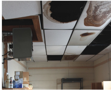
Facilities are in need of major operational and safety improvements.
