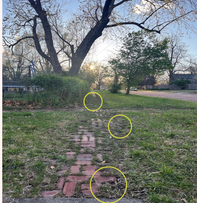
Category 5 – Vegetation overgrowth and protrusions
