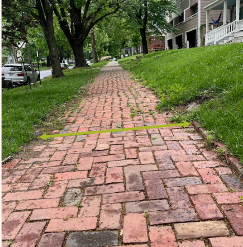
Category 4 – The sidewalk cross-slope exceeds 2%
