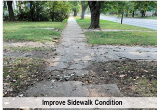
Improve Sidewalk Condition
