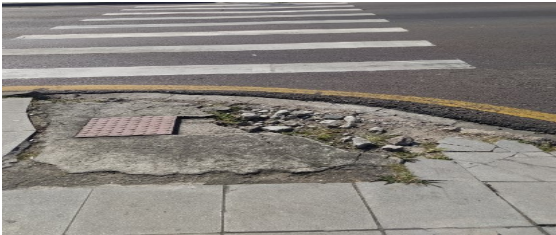
Figure 3: A Category 2 curb ramp with significant deterioration.
