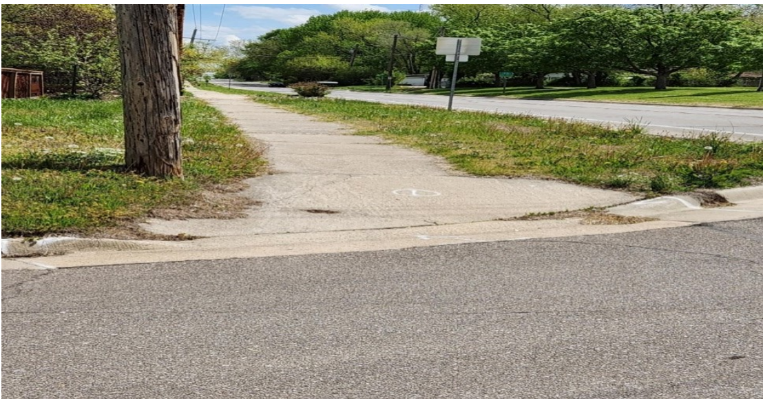
Figure 4: A Category 3 curb ramp with no detectable warning.
