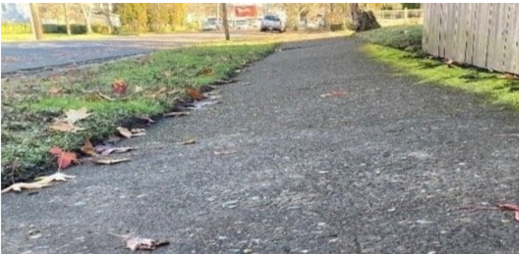
Figure 11: Sidewalk Category 4: the sidewalk cross slope exceeds 2%.
