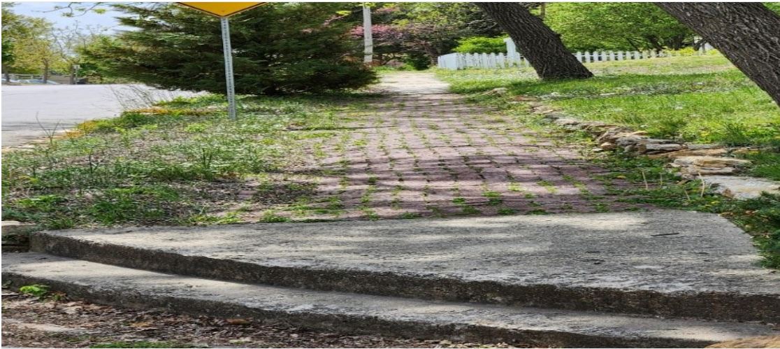
Figure 2: A Category 1 sidewalk with no ADA curb ramp present.
