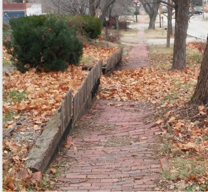
Figure 19: Brick sidewalk in poor condition.
