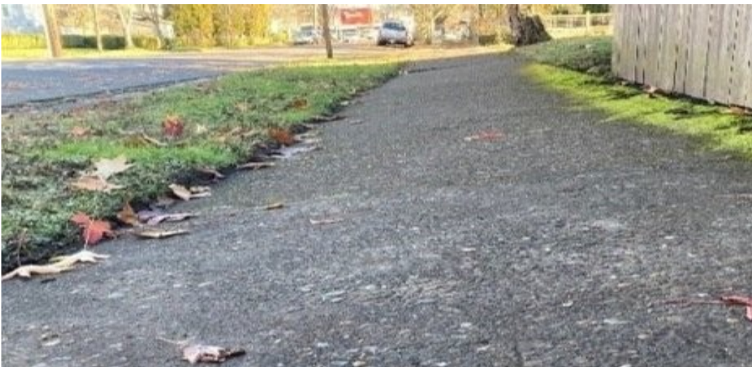
Figure 11: Sidewalk Category 4: the sidewalk cross slope exceeds 2%.
