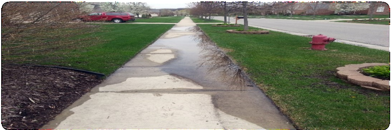
Figure 16: Sidewalk with excessive puddling
