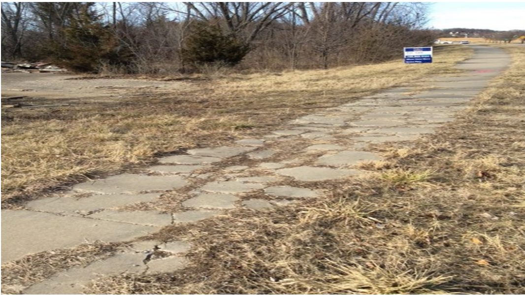
Figure 10: Sidewalk Category 3: the sidewalk is in poor condition, with multiple cracks and horizontal separations preventing access.
