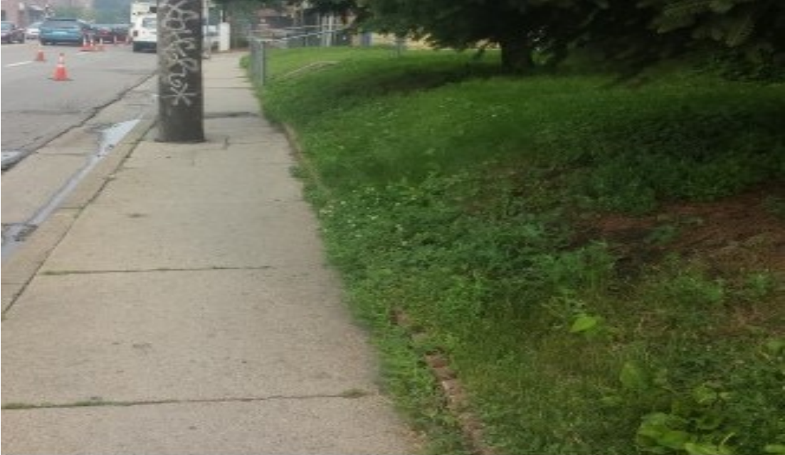
Figure 8: Sidewalk Category 1: the sidewalk is less than 48 inches wide.
